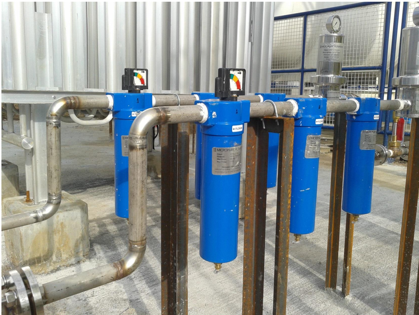
1 Inch SulfurGuard System with aluminum filter housings(stage V is stainless steel) 1,000 lb/hr of CO 2 flow
